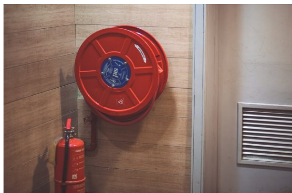
Figure 6. Fire extinguishers and hydrants
